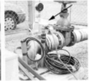
Deep well monitoring with Terminal box
